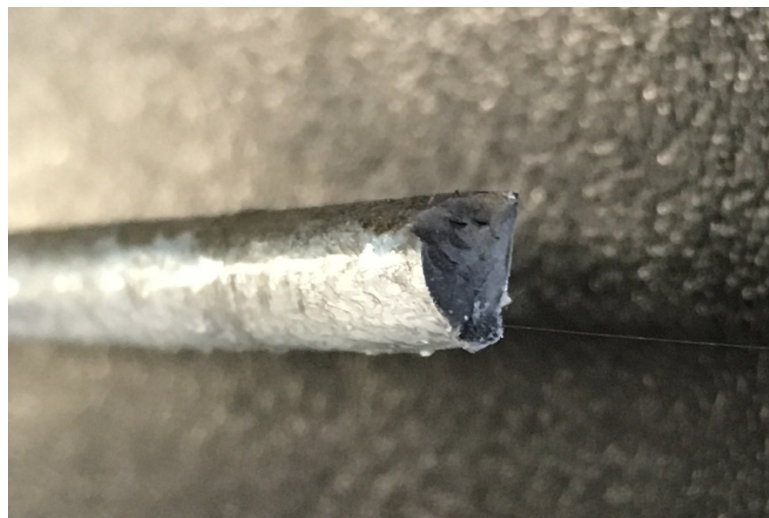
Figure 4.9. A wire fracture for S2.
