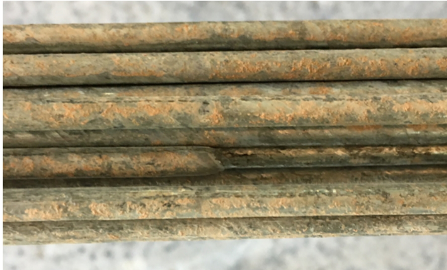
Figure 4.36. S5 discoloration and internal ruptured wire.
