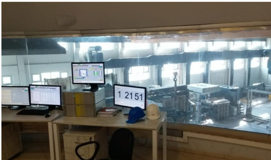
Figure 3.47. The view of the furnace control center from TSE Laboratories Complex.
