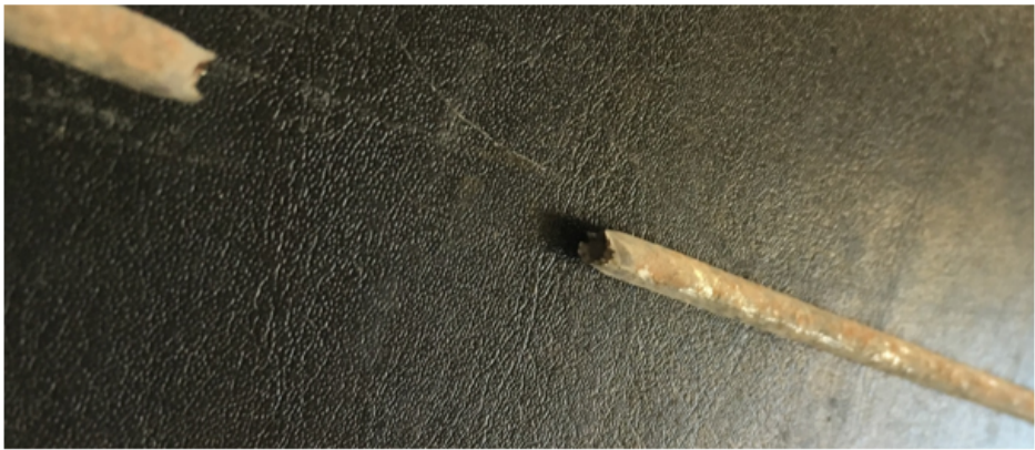
Figure 4.39. A wire fracture for S5.
