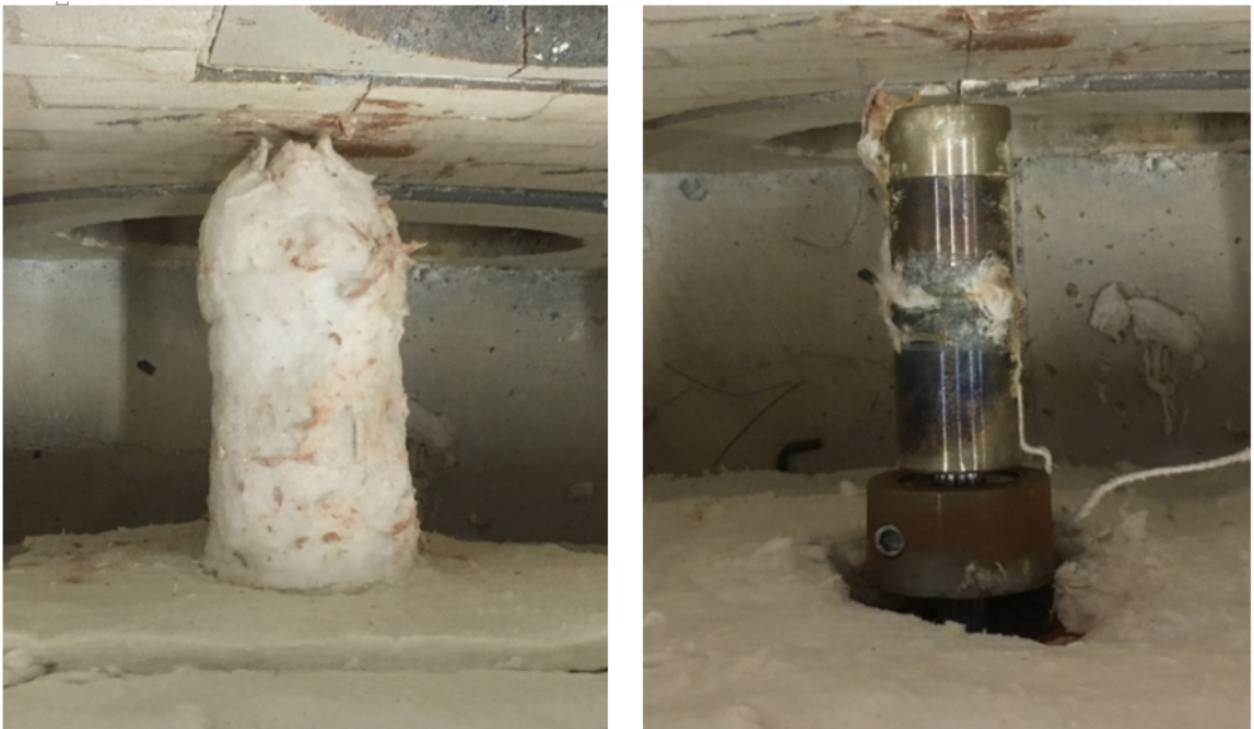
Figure 4.30. S5 socket protection prior to fire test and S5 socket condition after fire test 5.
