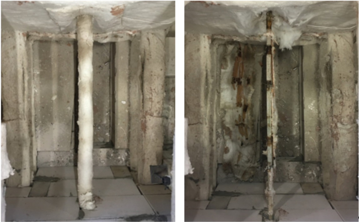
Figure 4.29. S5 strand protection prior to fire test (left-hand side) and S5 condition after fire test 5 (right-hand side).
