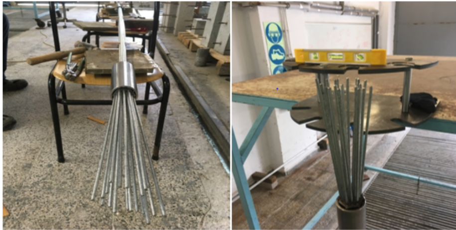
Figure 3.24. Preparation for socketing (left-hand side), prior to clamp the wires on socket holding system (right-hand side).
