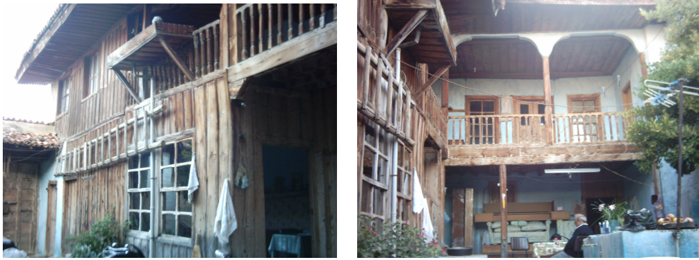
Figure 80, Case 8, View of the residential unit from the courtyard and service spaces on the ground floor (Taşdöğen)
