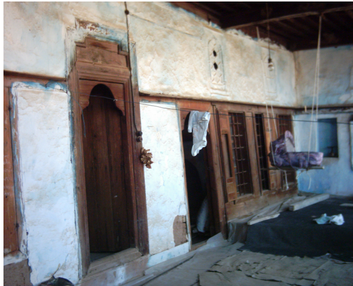
Figure 89, Case 10, Hayat and the rooms opening to hayat on the first floor (Taşdöğen)
