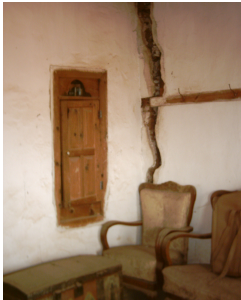
Figure 62, Case 3, Crack on the wall of a room upstairs (Taşdöğen)
