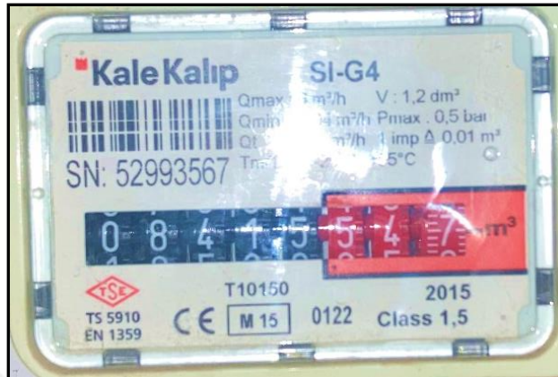
Figure 5.2 Natural gas cubic metering before third condition test (Personnel Archive, 2023)
