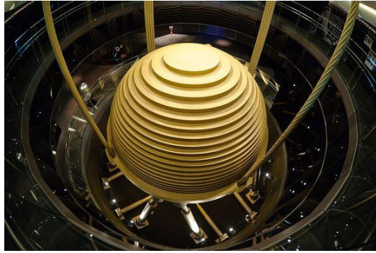
Figure 1.6: Tuned mass damper
