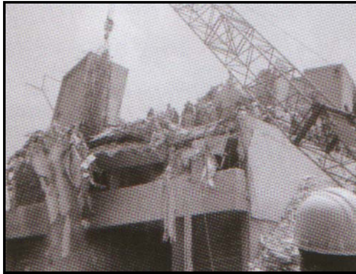
Figure 3.12 Collapsed building in downtown Mexico City
