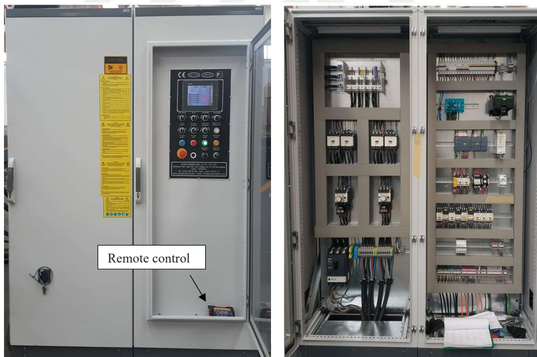
Figure 1.14 Electric-automation board (Personal archive, 2019)
