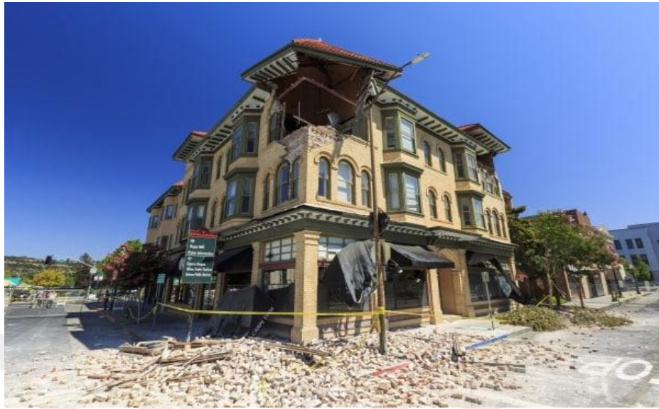
Figure 2.11 The earthquake damage to this building may have been influenced by the type of soil it's sitting on. (Nolan, 2022)
