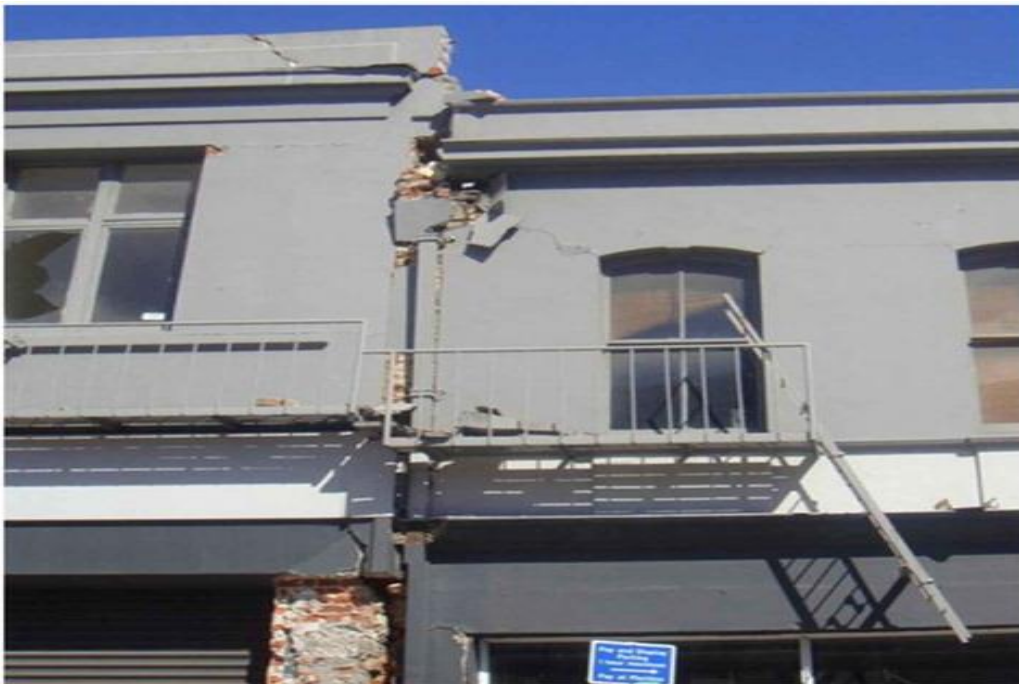
Figure 4.27 Pounding damage observed in Christchurch CBD, 2011 (Noman et al., 2016)
