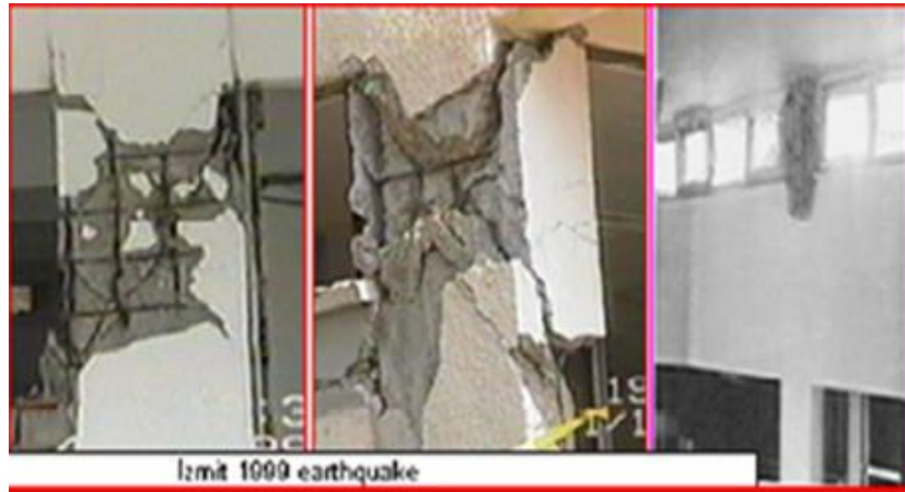
Figure 2.9 Examples of short column failures observed after earthquakes (Isik, 2006)
