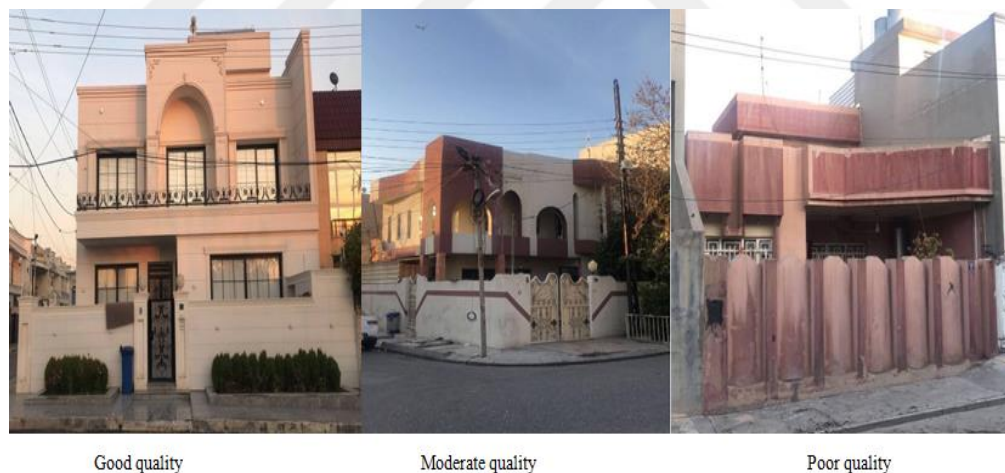
Figure 4.22 Shows three types of apparent building quality in Brayaty Quarter in Erbil City
