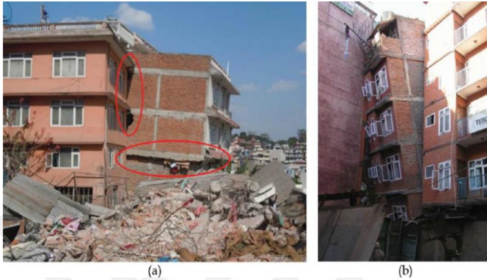
Figure 2.5 (a)The intermediate storey collapsed due to the adjacent building pounded against it, and (b) collapse due to extension of the upper storey plan beyond the column grid lines which created vertical irregularity
