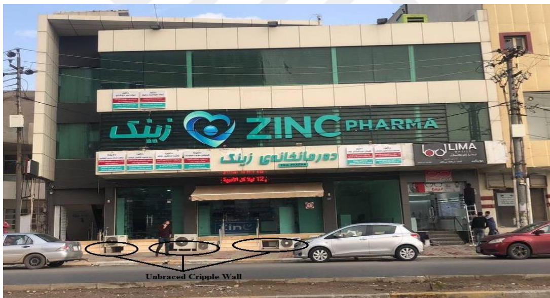
Figure 4.10 Unbraced cripple wall in the building in Brayaty Quarter in Erbil City
