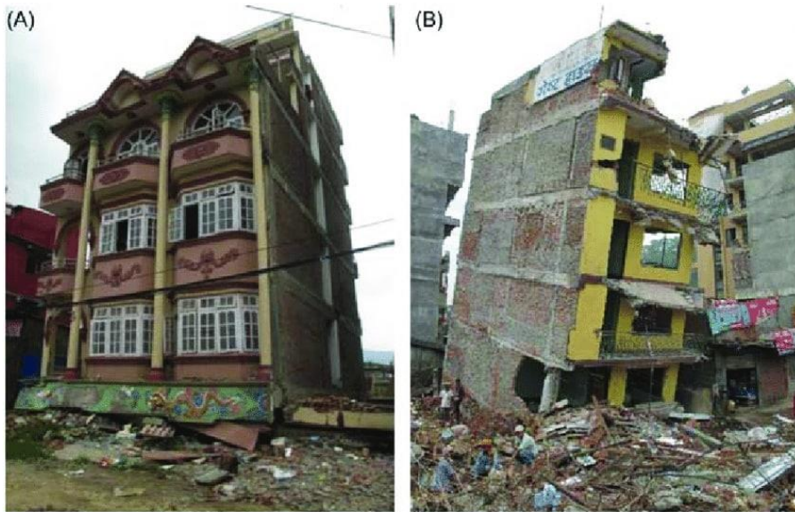
Figure 2.2 Examples of Nepal earthquake-related buildings that experienced soft-story collapse
