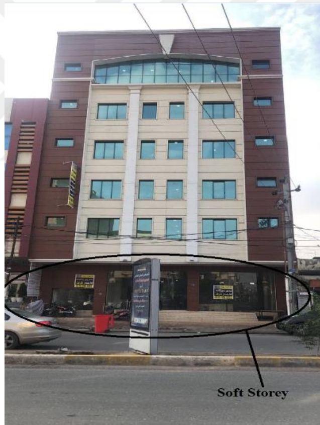
Figure 4.20 Illustrates presence of a soft storey in the building in Brayaty Quarter in Erbil City
