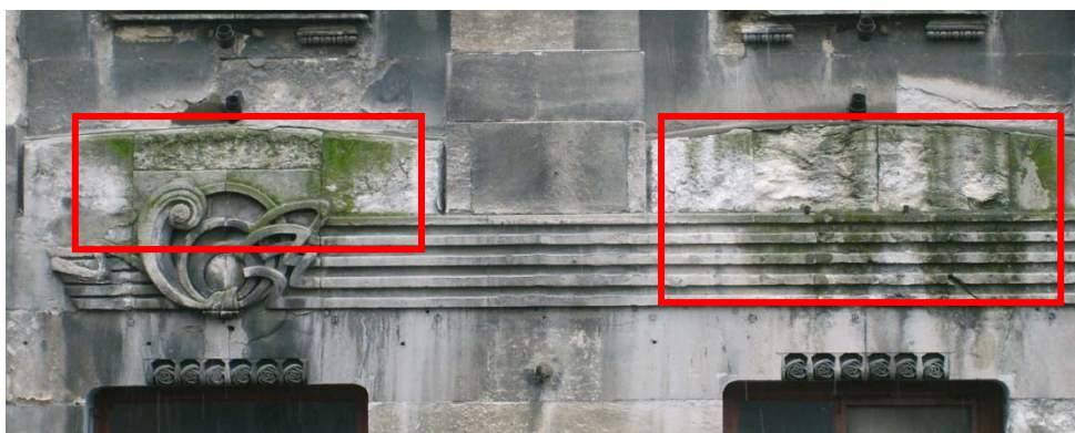
Figure 28. Microbiological Colonization on the façade of the Botter Apartment
