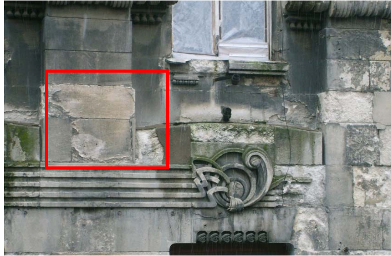
Figure 31. Scaling on the façade of the Botter Apartment
