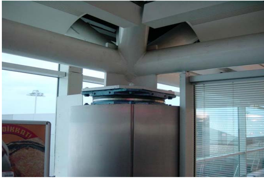
Figure 6.25. Location of a FPS isolator in Atatürk Airport
