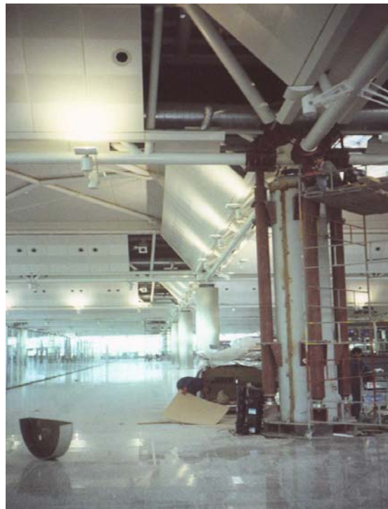
Figure 6.24. Locations of FPS isolators in Atatürk Airport
