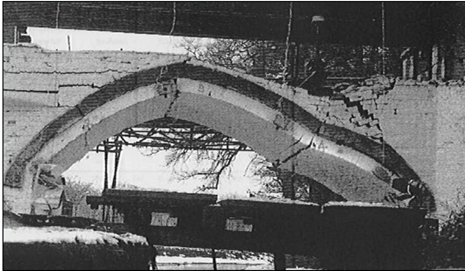
Figure 3.12. Collapse of Prestwood Bridge [35]
