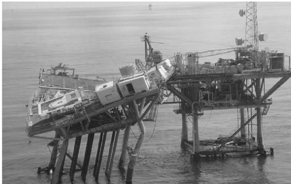
Figure 1.1 : An offshore platform sustained significant damage during a hurricane near louisiana in the gulf of mexico.
