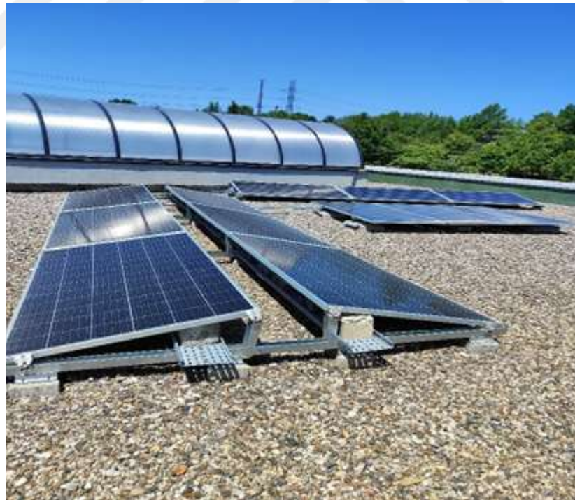
Figure 4.1. PV rooftop system at M6 building.
