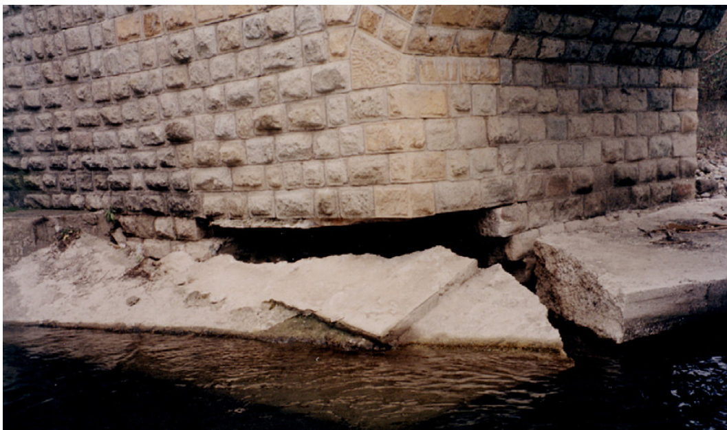
Figure 3.10 Substructure failures due to settlement problems on the Mataraci Bridge (Ural et al. 2008)
