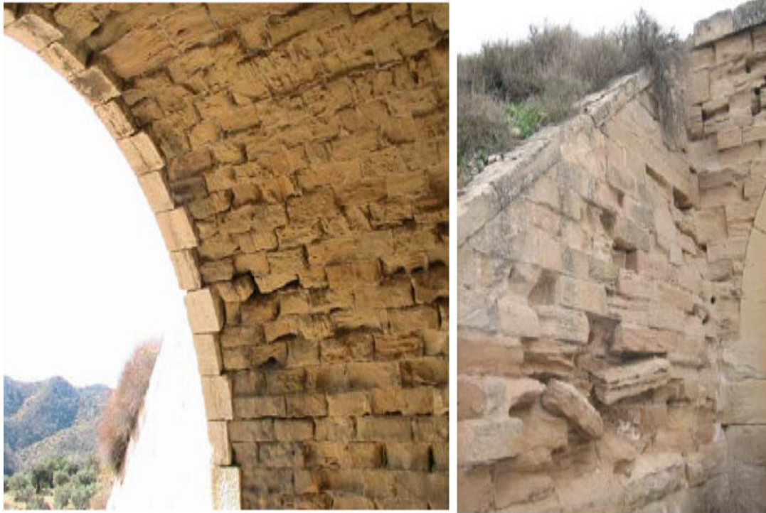
Figure 3.14 Deterioration of construction materials (Catalán and Álamo 2006)
