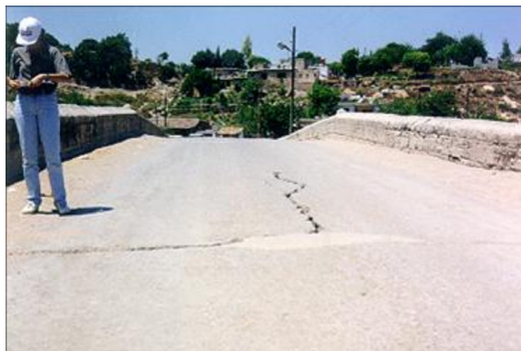
Figure 3.7 Damages occurred in superstructure of the Misis Bridge during the 1998 Adana-Ceyhan earthquake (Ural et al. 2008)
