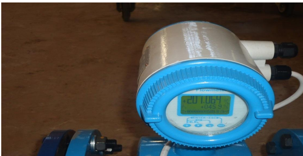
Figure 3.2. Magnetic flow meter installed in the pipe system
