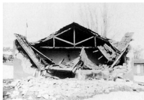
Figure 5.11 from the top-down: a heavily damaged traditional building in the village of Altınbaşak; a damaged adobe brick infill wooden frame house in the village of Altınbaşak; a collapsed single-storey adobe and clay brick masonry house in the village of Yalnızbağ; and a collapsed stone masonry school building in the village of Mecidiye (Williams et al., 1992).
