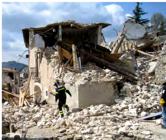
Figure 2.23 A totally collapsed unreinforced stone masonry building in Castelnuovo village (Lanzo et al., 2010).
