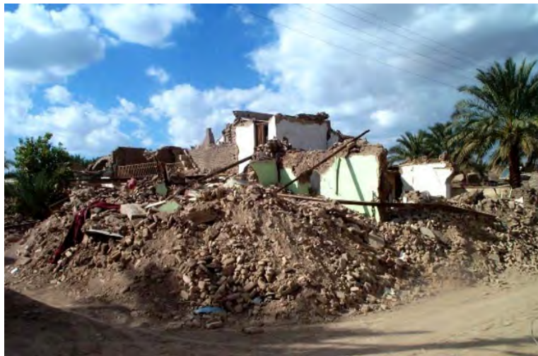
A totally collapsed adobe masonry building, Bam, Iran (Manafpour, 2008).
