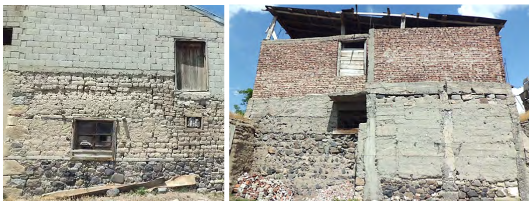
Figure 3.13 An example of a barn with faulty extended wall and a two-storey house, of which the second floor is added on the stone masonry ground floor with discontinuous concrete ring beam and columns.
