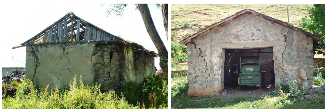
Figure 3.12 An example of masonry structure poorly built with rubble stone and an example of a masonry structure built with cement mortar that is used as a garage; both suffer large cracks in the corners.
