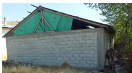
Figure 11 from top-down: a view of a damaged house since 1992; the house built in the opposite of the ruin; a barn built by a dweller.
