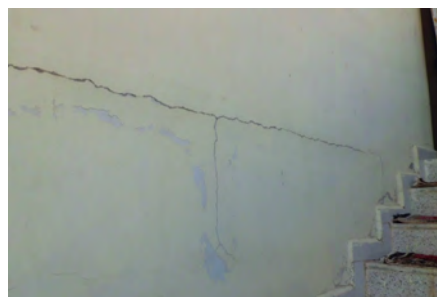
Figure 7 from the top-down: a porch built with different materials added to the entrance of a two-story house; an extension built under the cantilever and the entrance; view of exterior stairs of an unoccupied building; and cracks on an exterior wall by the entrance.
