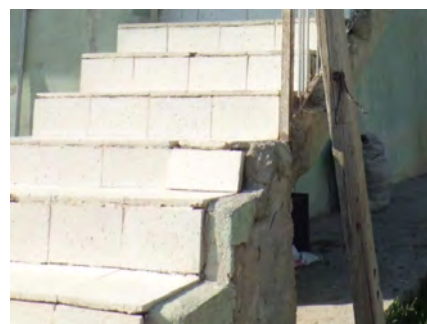
Figure 10 from top-down: the satellite view of Tazegul; the abstract map shows the locations of the post-earthquake permanent houses built in the former and the relocation site; a view from a two-story house; and, a view from the stairs poorly constructed.
