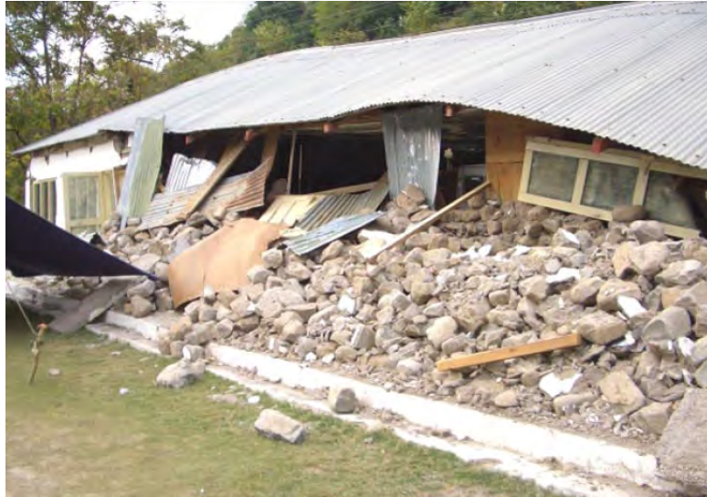
A collapsed stone masonry house, Kashmir, Pakistan (EERI, 2005)
