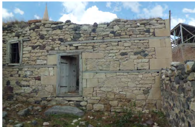
A traditional stone masonry building abandoned and half collapsed.
