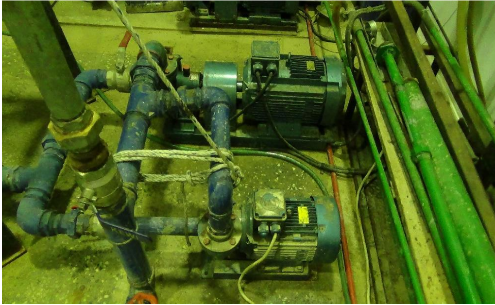
Figure 3. 10 Centrifugal Pumps for Circulating the Fluid through the System
