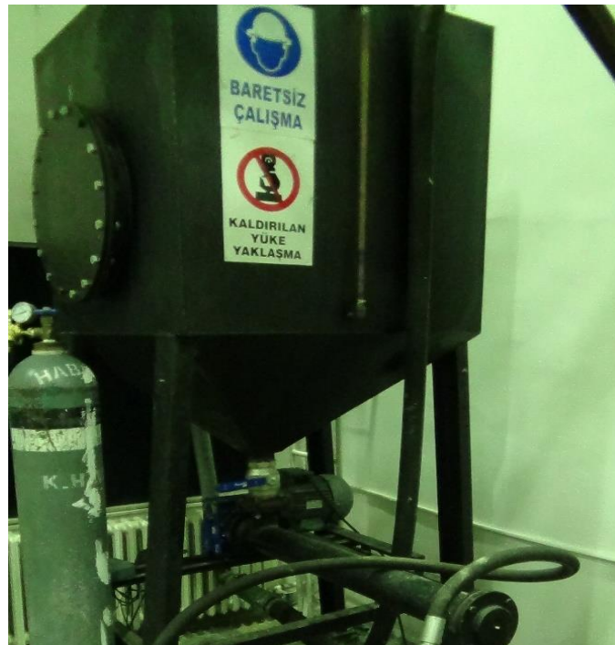
Figure 3. 7 Cuttings Injection Tank
