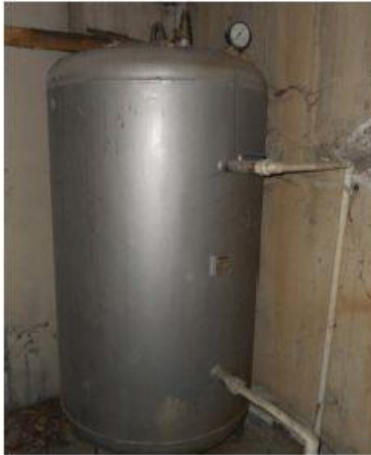
Figure 3. 14 Air Accumulator Tank
