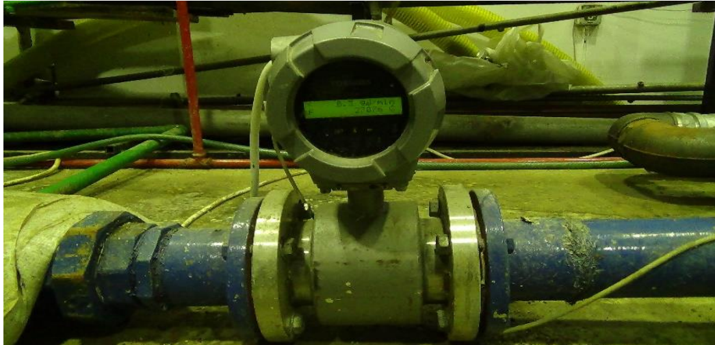
Figure 3. 12 Toshiba Flow Meter
