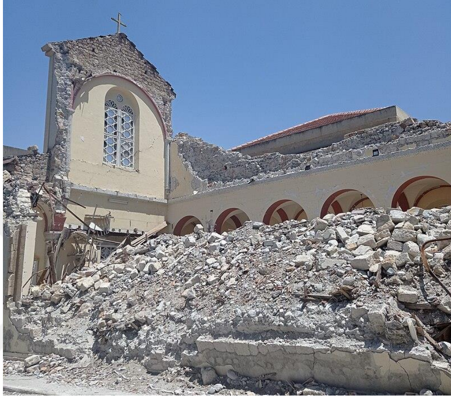
Figure 5.3. The Cathedral of Iskenderun (Alexandretta) destroyed by 7.7 magnitude earthquake [101].
