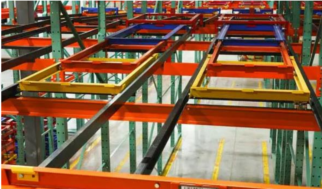
Figure 4. Push back pallet rack .
