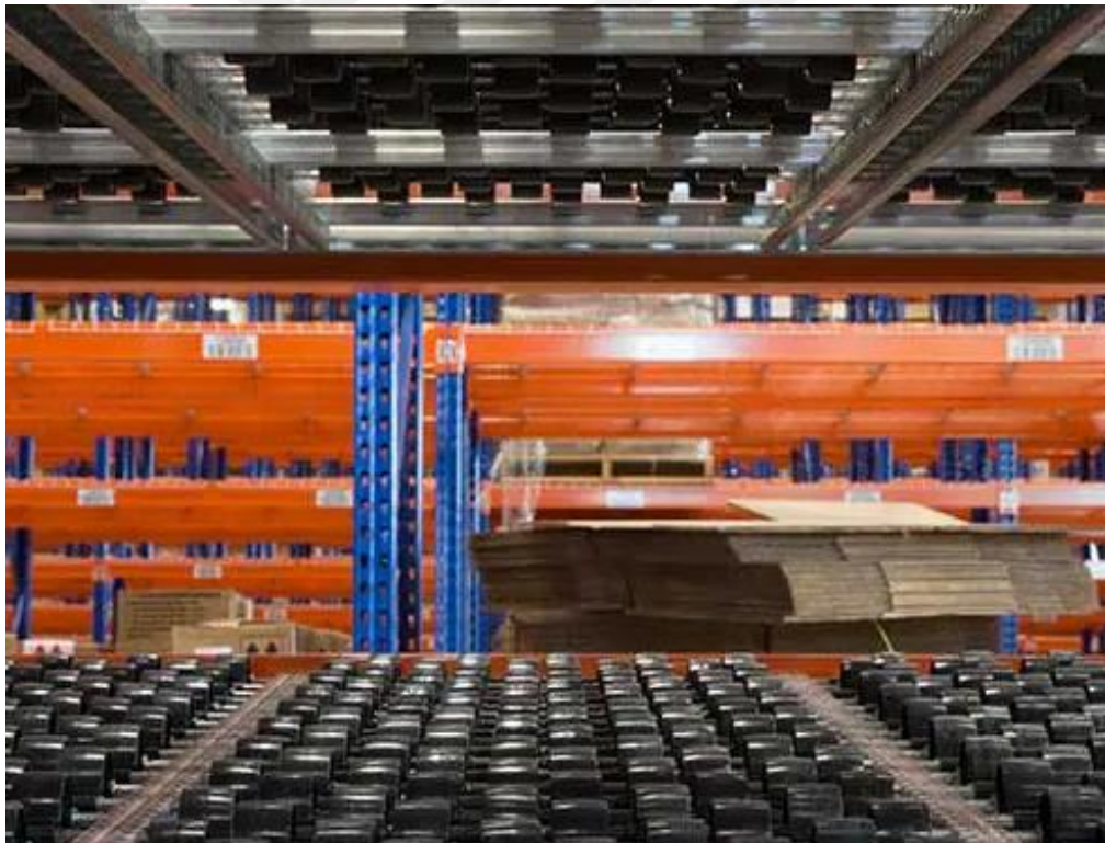
Figure 6. Flow racking system .
