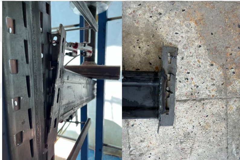
Figure 51. Failure mode A+B (deformation of beam end connector and deformation of tabs).
