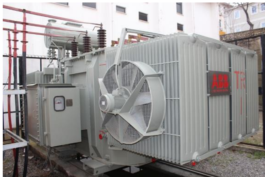
Figure 9: Tank with Radiator
