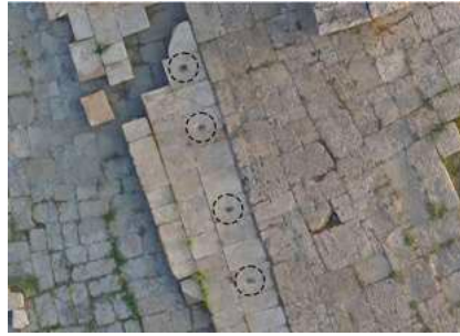
Figure 35: Cavities formed due to abrasion of rings.
