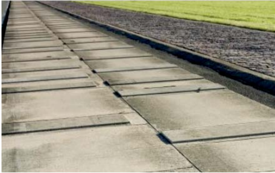
Figure 8: Resonance Road Surface [39]
