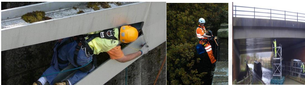
Figure 1.2 Risky conditions in building inspection
