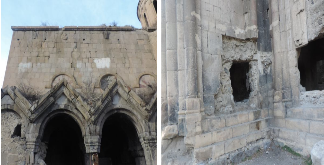
Figure 4.10: Some Cracks Observed on the Exterior Facade of the Structure.
