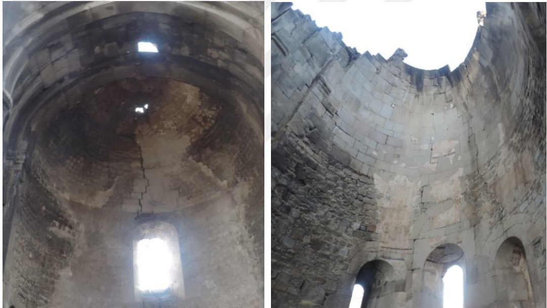
Figure 4.11: The Damaged Dome and Apse Section on the Interior Facade of the Structure.
