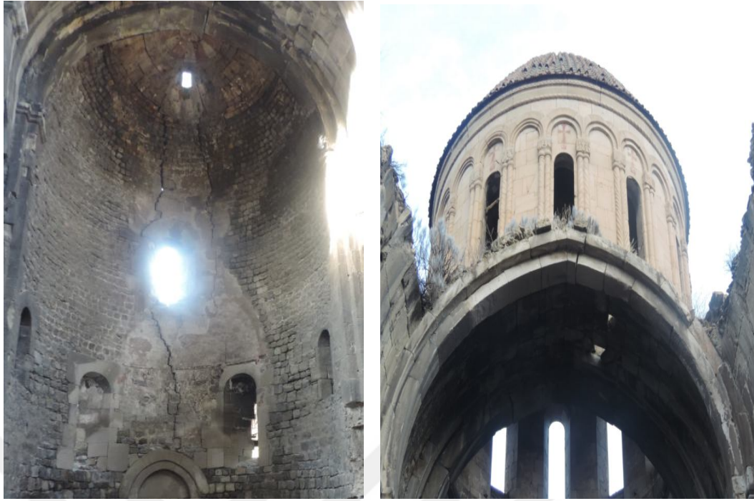
Figure 4.12: Some Damages Observed on the Interior Facade of the Structure.
