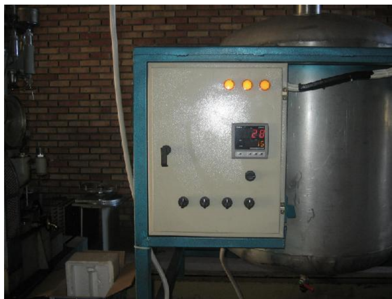
Figure 3.6. Control Panel (ETC 942).
