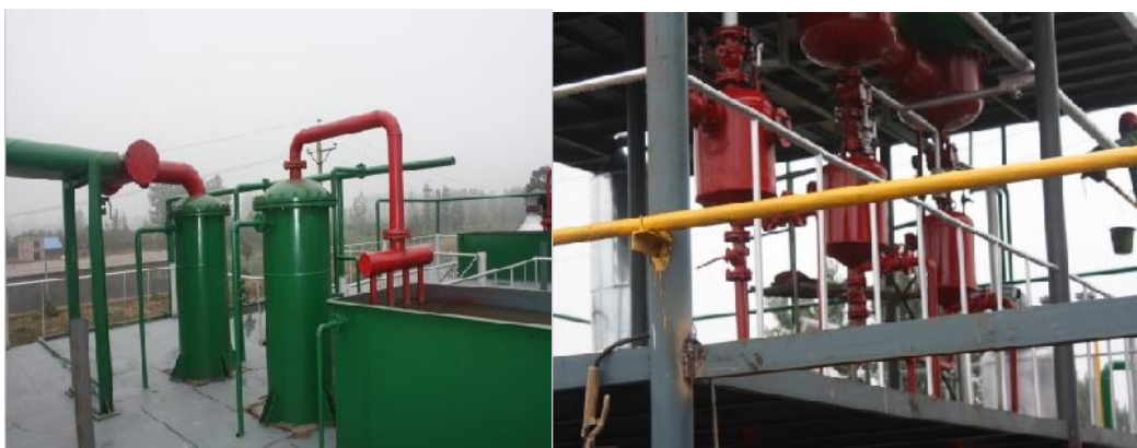
Figure 3.17. Condensers and spray cooling pipes.
