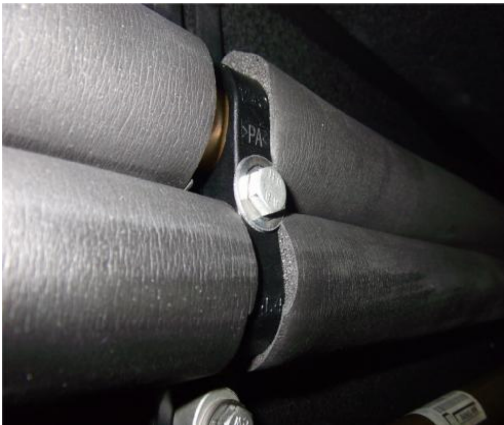
Figure 4.13. Insulation for the piping to the heaters, the bracket ist made of plastic
