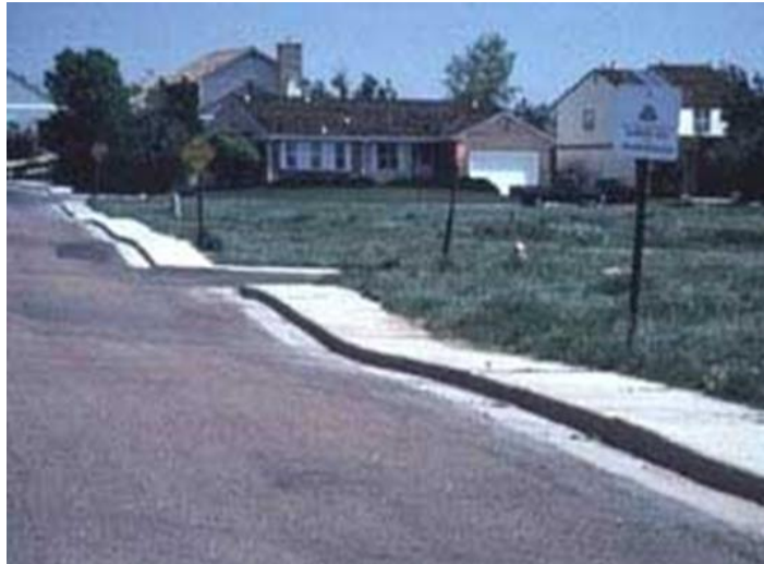
Figure 1.3 A view of road undergoing swelling
