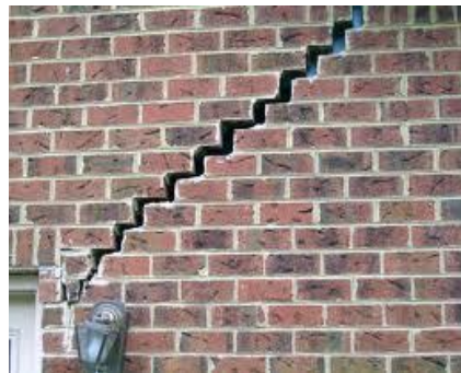
Figure 1.2 Damage on a masonry wall due to the shrinkage in Soil ( www.basementsystems.com , 2016)
