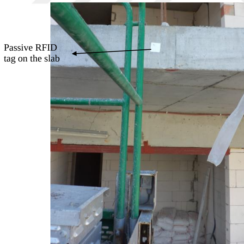
Figure 4.11 : RFID tag on the floor slab.
