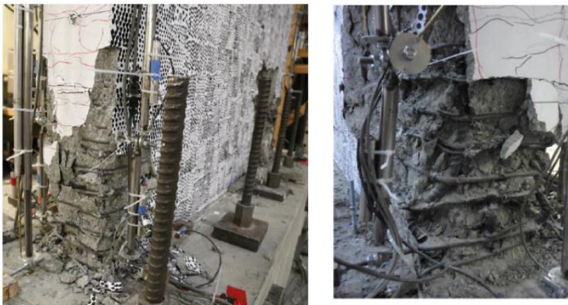
Figure 3.21 : Segura (2017) – WP7 west and east boundary final damage state.
