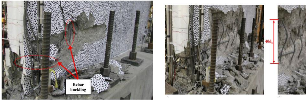
Figure 3.17 : Segura (2017) – WP3 east and west boundary final damage state.
