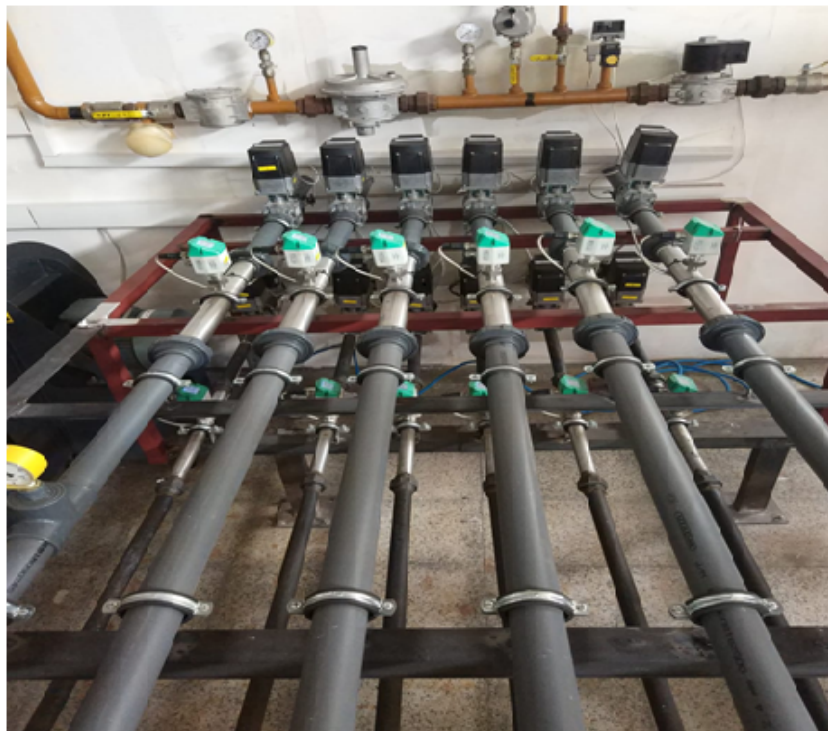
Figure B.2 : Air and natural gas pipeline.
