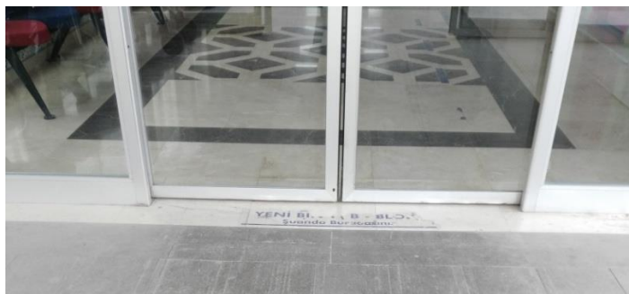
Figure 4.33. Wide enough entrance but not having tactile surfaces
