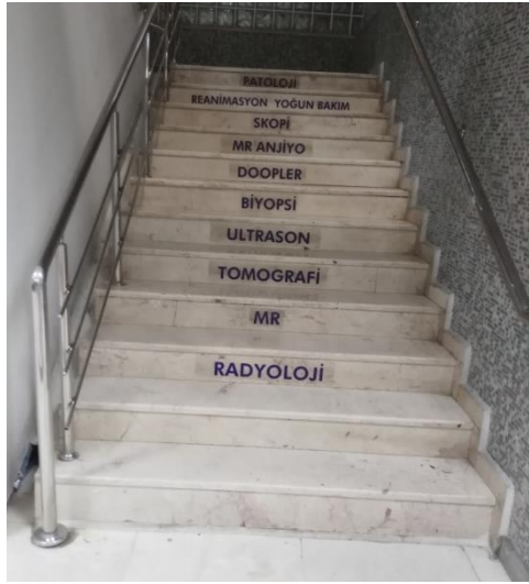
Figure 4.34. Stairs not having tactile surfaces and slip-resistant strips
