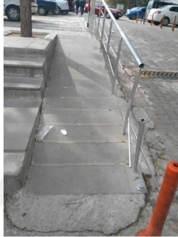
Figure 4.31. Upright ramp having broken handrail and not having tactile surfaces
