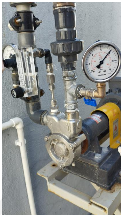
Photo 3.5 Piping of the MB-DAF-1 System (Personal archive, 2022)
