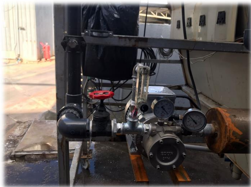
Photo 3.7 Piping of the MB-DAF-2 System (Personal archive,2022)
