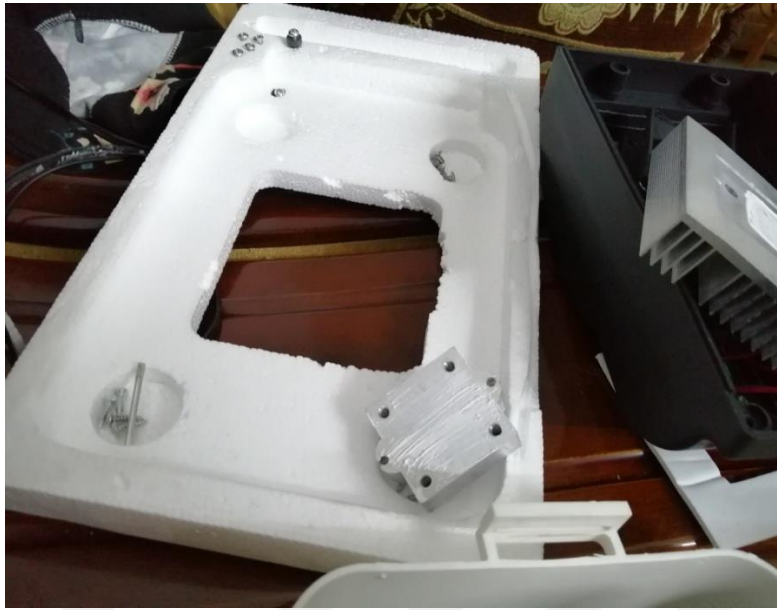
Figure 3.10: Cutting a space for Peltier module in the thermocol wall of the box
