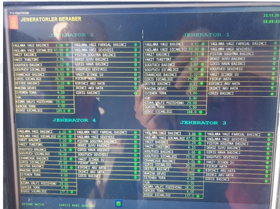
Figure 1.6 : Diesel generators control panel.
