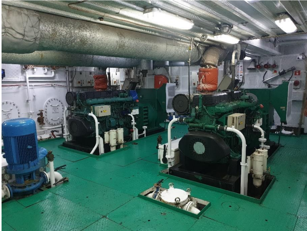
Figure 1.4 : Part of engine room of the case ship.
