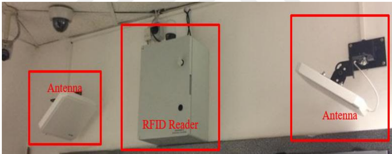
Figure 27 RFID Reader and Antennas Location
