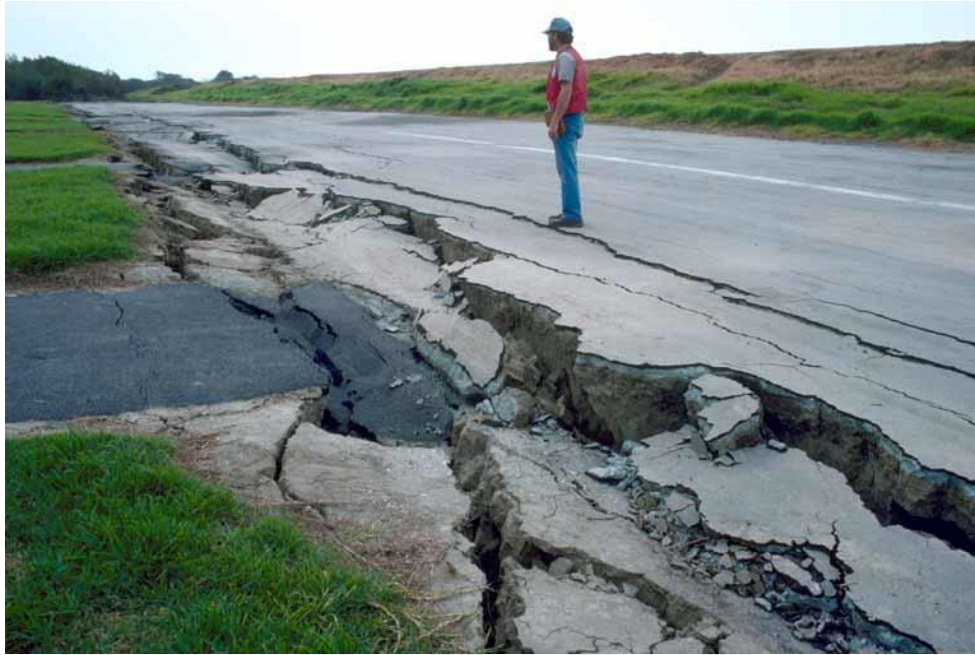
Figure 2.15. Lateral spreading (Source: wikipedia).
