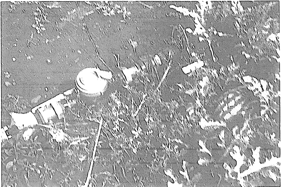
Figure 2.5 Water-meter used in the drip irrigation system
