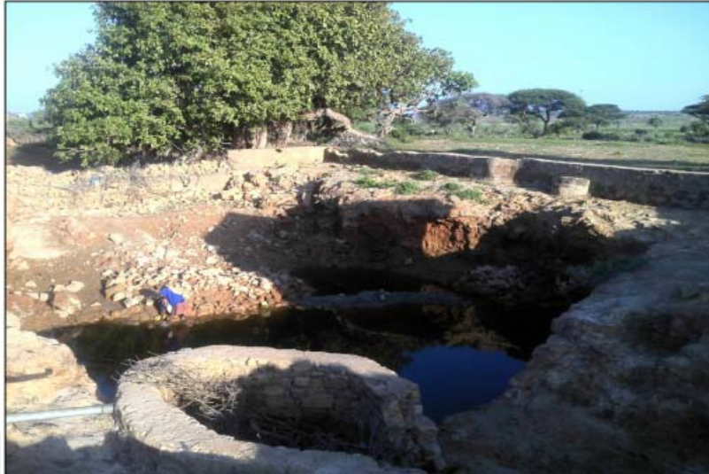
Figure 5. 1. Sink hole (unprotected) of Godalo area (SHAAC, 2010)
