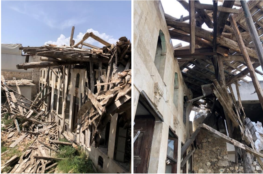
Figure 2.51 First floor failure (METU TAÇDAM, 2023)
