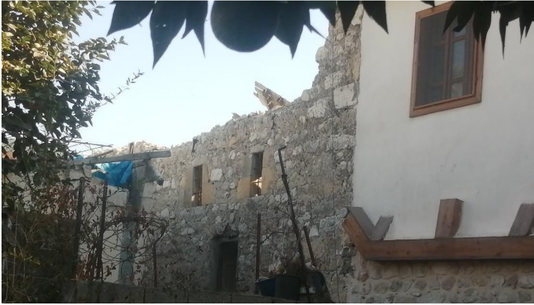
Figure 4.1 Out-of-plane collapse of the north wall on the first floor
