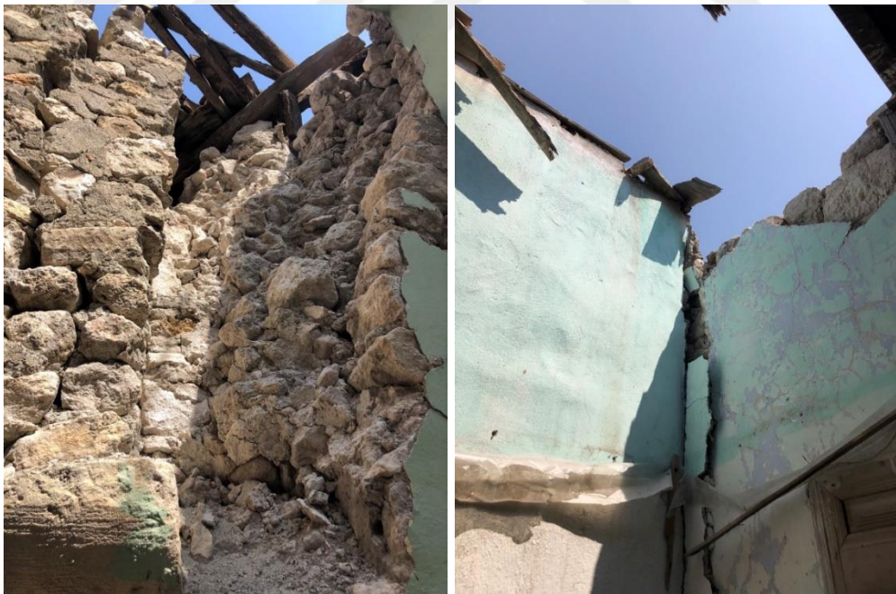
Figure 2.52 Wall coursing with weak mortar (left) and wall intersections (right) (METU TAÇDAM, 2023)
