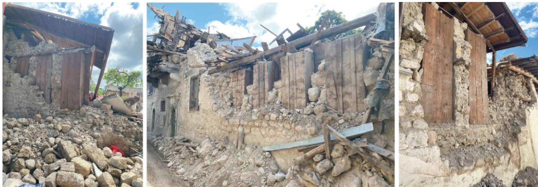
Figure 4.10 The superior performance of niches and timber frames embedded into masonry walls during the 2023 earthquakes (Rifaioğlu et al. 2024)
