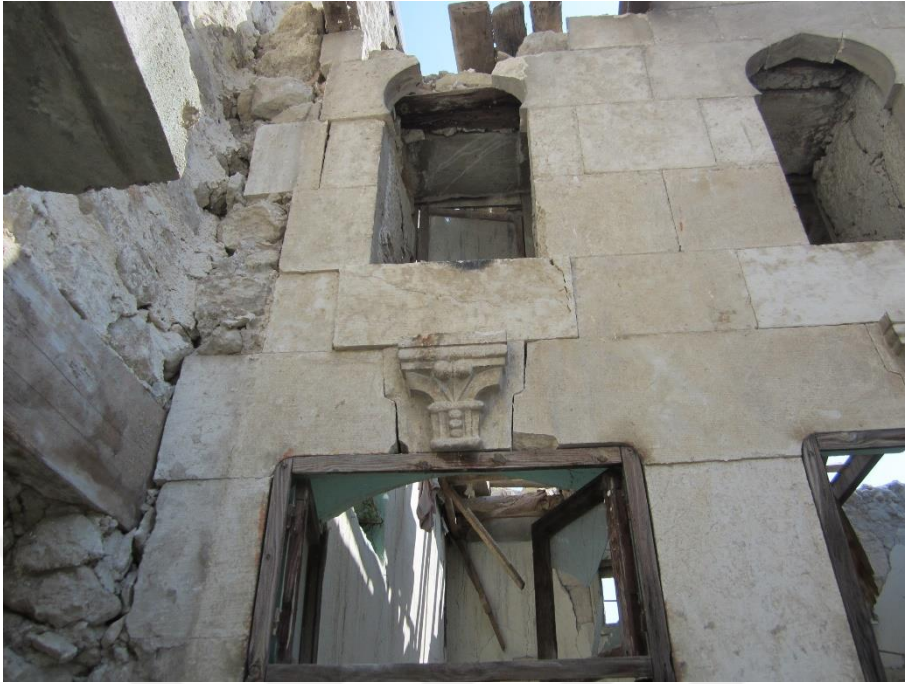
Figure 4.8 Observed damage in the upper corner of the openings in the south wall of the ground floor (METU TAÇDAM, 2023)
