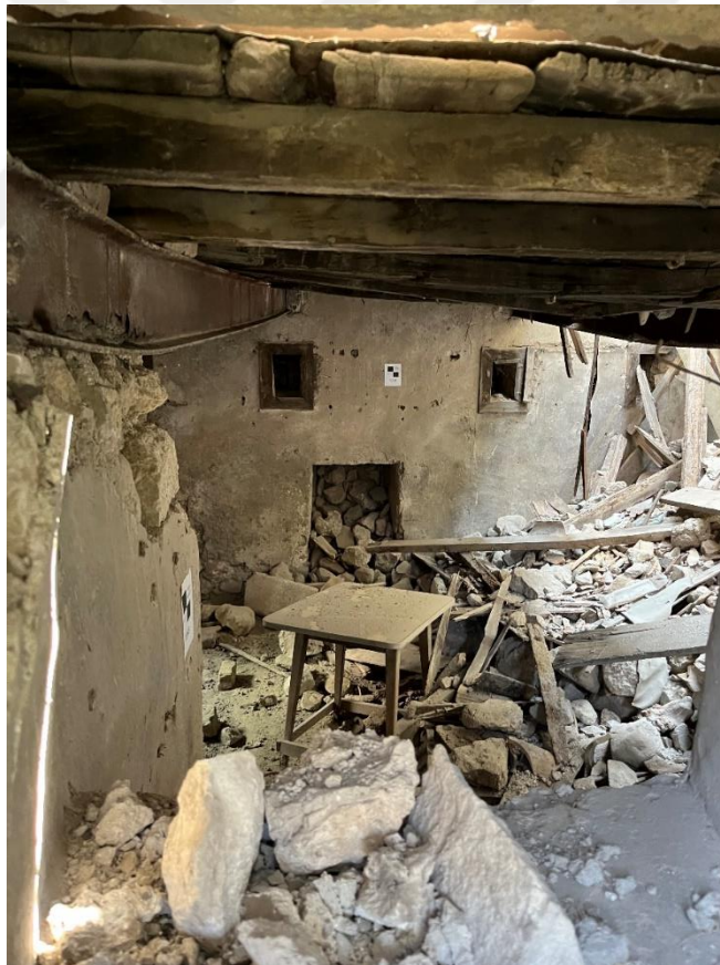
Figure 2.50 Damage in the B01 room (METU TAÇDAM, 2023)
