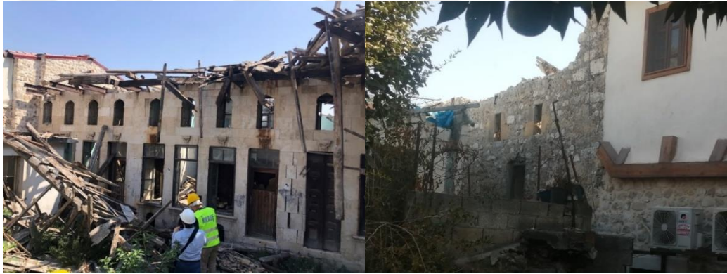
Figure 2.48 South and north wall (METU TAÇDAM, 2023)
