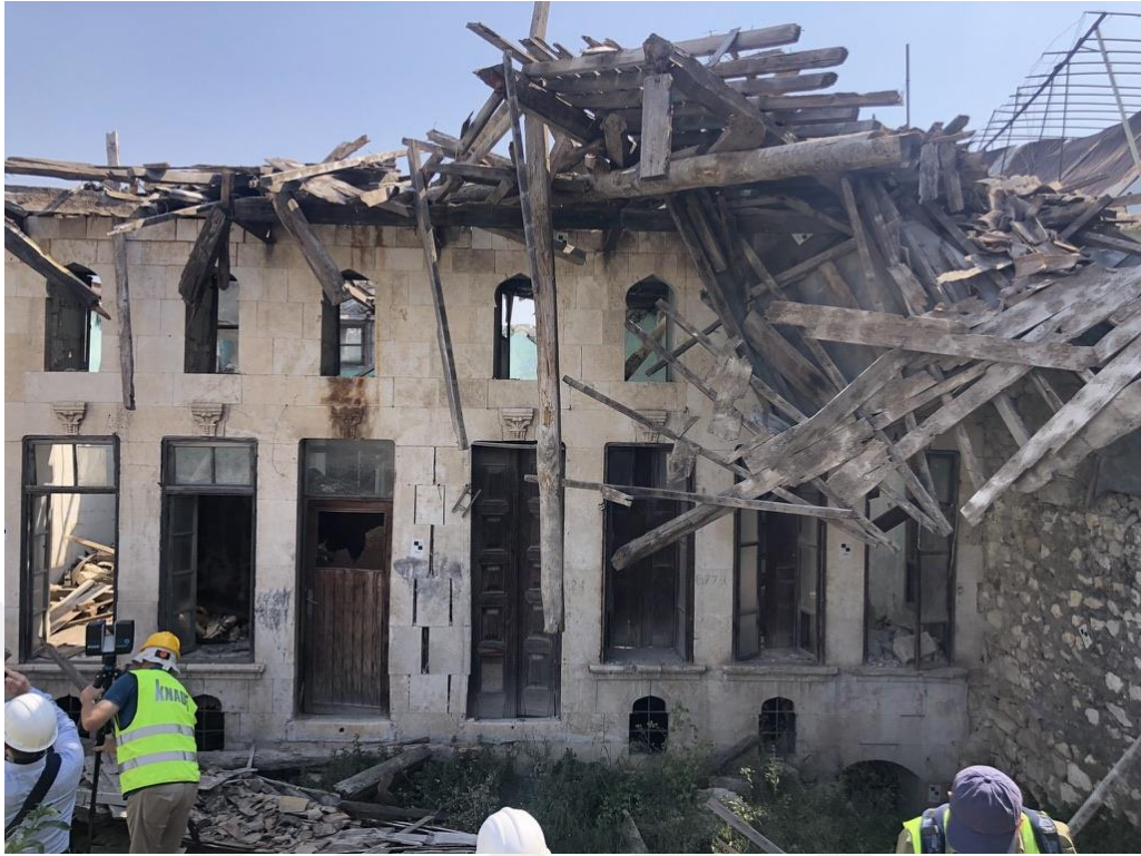
Figure 4.6 Observed earthquake damage for the south wall (METU TAÇDAM, 2023)
