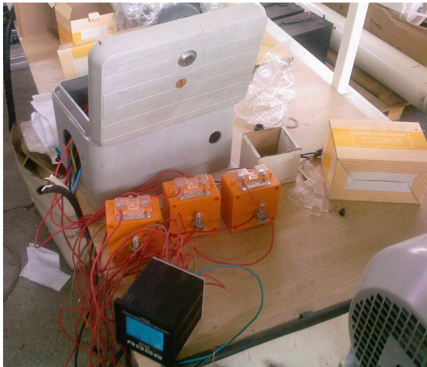
Figure 67 Energy Analyzer for Power Measurement
