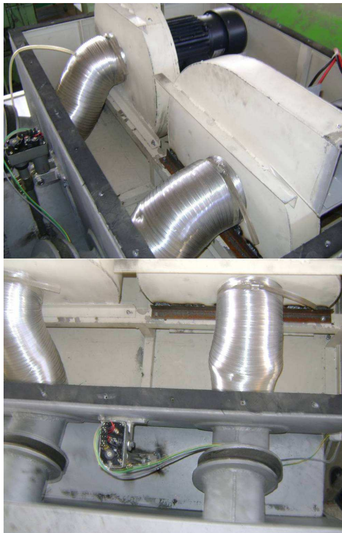
Figure 96 Views of Connection of the Fans Directly
