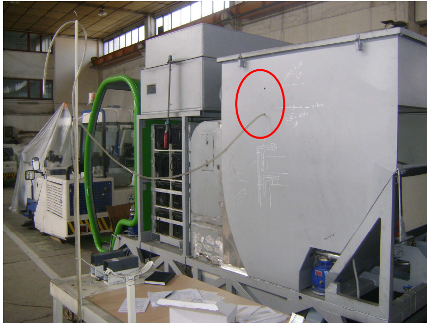
Figure 94 'U' Manometer and Drilled Measurement Holes
