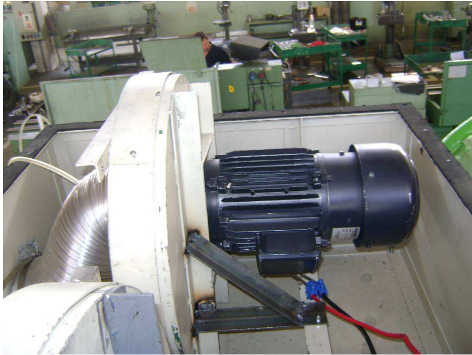
Figure 97 Electric Motors and Fans
