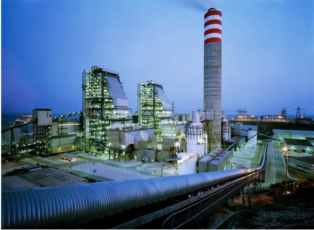
Figure 3.4. The steam power plant
