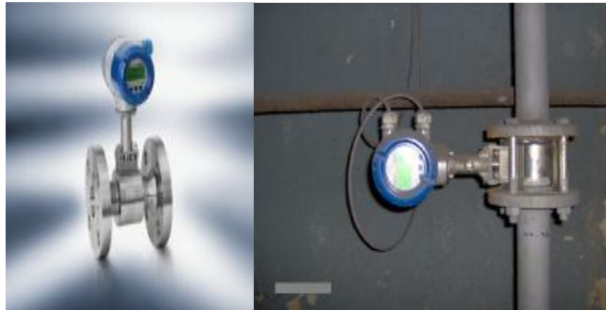
Figure 6.1 General overview of flowmeter and device on line.
