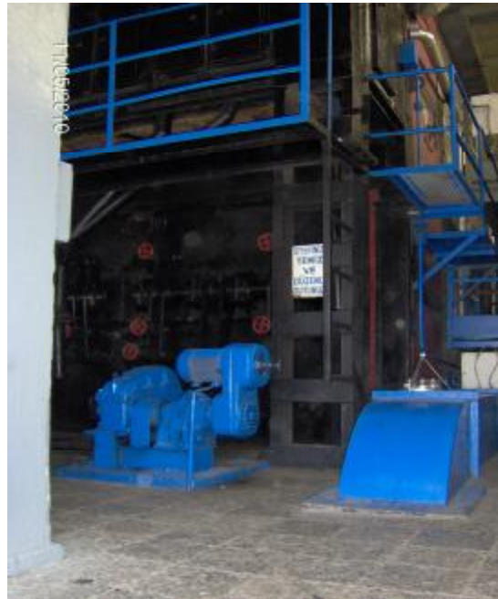
Figure 4.7 An overview of coal fire boiler of MARSAN A.Ş
