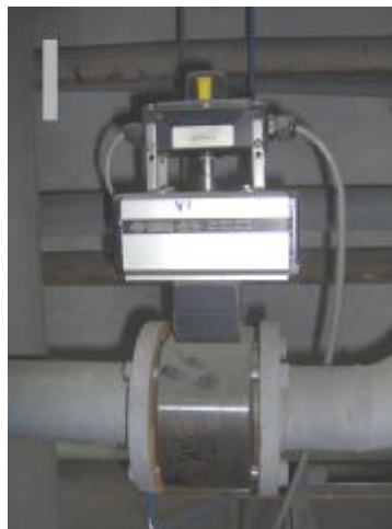
Figure 6.2 DA 120 F05-F07 OMAL on/off ball valves mounted on system
