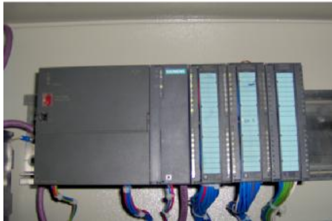
Figure 6.10 Deodorization plant side. Control system of project
