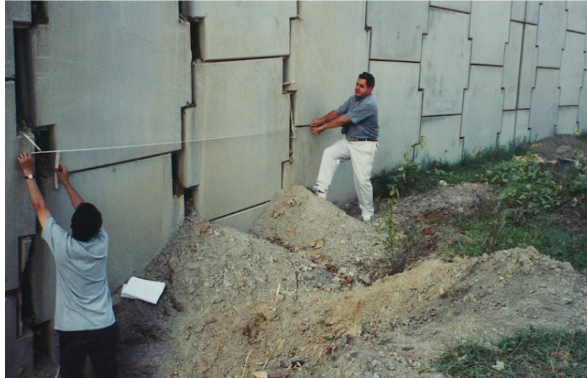
Figure 5.4 : The 1999 kocaeli earthquake in turkey, Reinforced earth MSE wall (Reinforced earth company, 1999).
