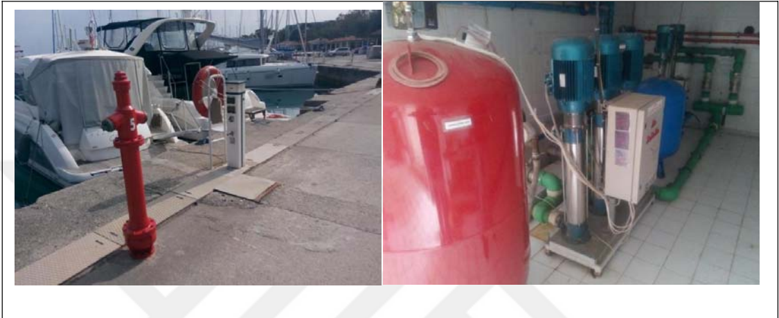
Image 13. Sea Water Pipe and Pressurized Sea Water System
