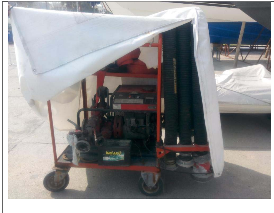
Image 12. Portable Fire Pump in T Marina
