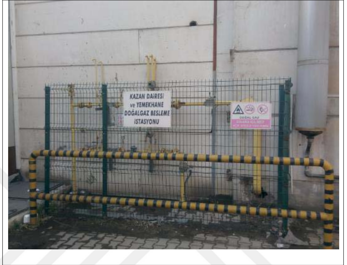
Image 10. Natural Gas Pipe Line in R Port
