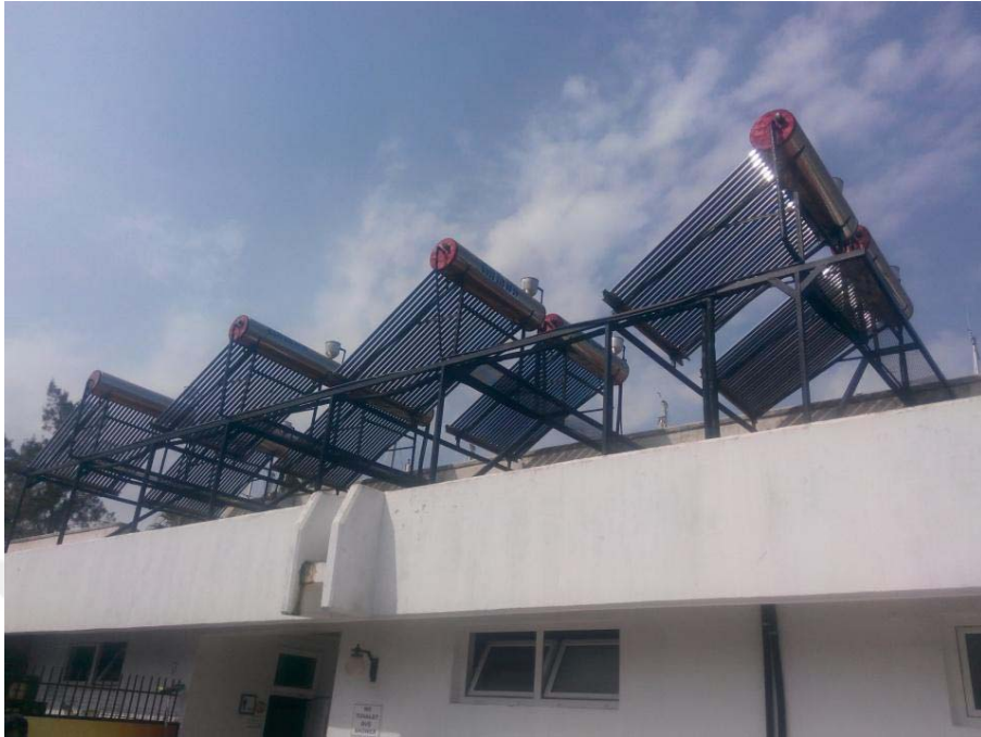
Image 8. Solar Energy Station For Water Heating In T Marina
