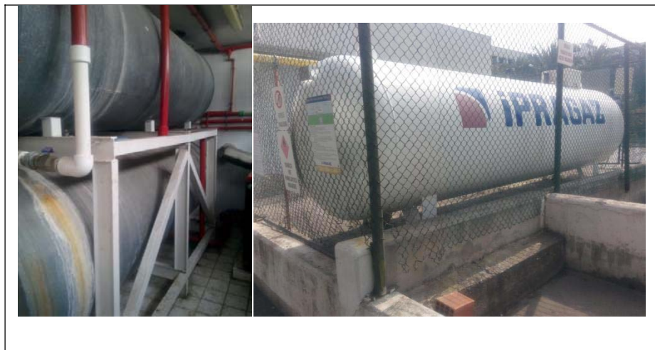
Image 9. Natural Gas Facilities in T Marina
