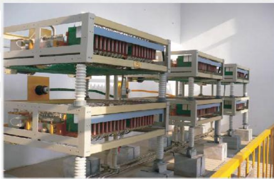
Figure 4.17 Thyristors valve of SVC
