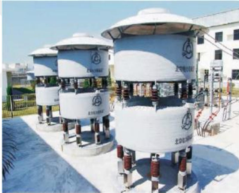
Figure 4.21 TCR reactor of SVC
