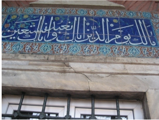
Figure 5.11: Cracks of window edges
