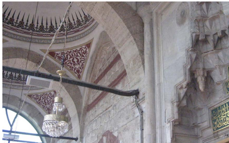
Figure 5.12: Buckling damage of iron ties.
