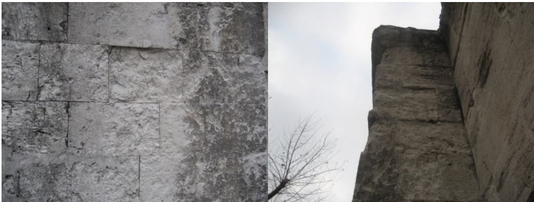
Figure 5.10: Stone deterioration on the wall of the cloister.
