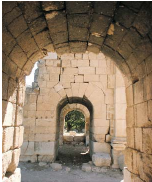
Figure 4.5: Pointing separation of the vault (Sesigür et al., 2007).
