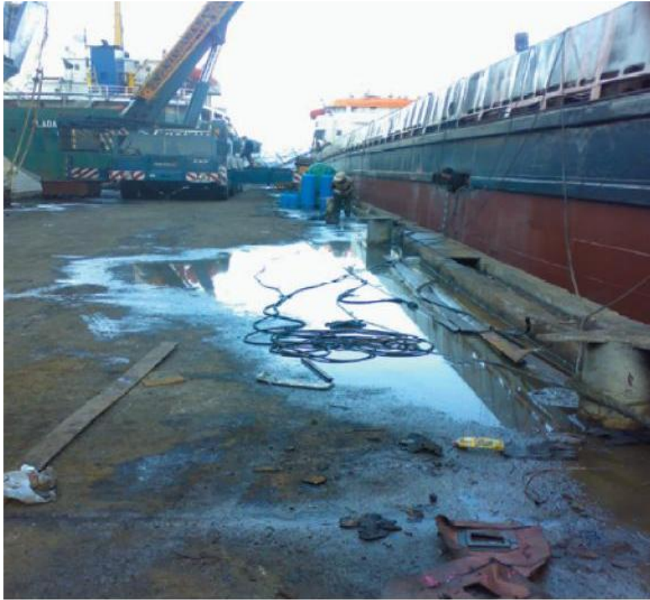
Figure A.3. Damaged Electric Cables over Wet Floor (TMLSS, 2007)
