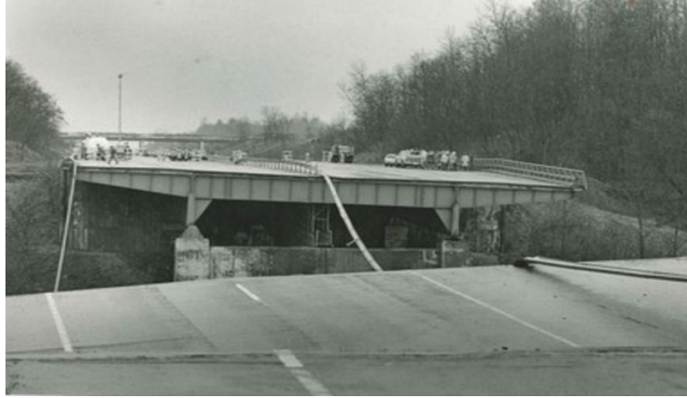
Figure 1.3 Eastbound view of the New York State Thruway bridge collapse over the Schoharie Creek on April 5, 1987.
