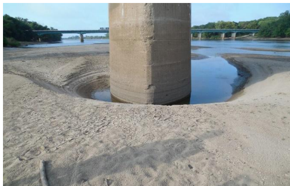
Figure 1. 1 Scour hole around bridge pier (Melville & Coleman, 2000).
