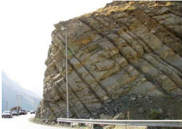
Figure 1.1 Example of rock blocks exposed to toppling failure
