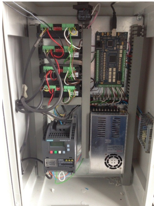
Figure 4.25 Electrical cabinet of motion control system.
