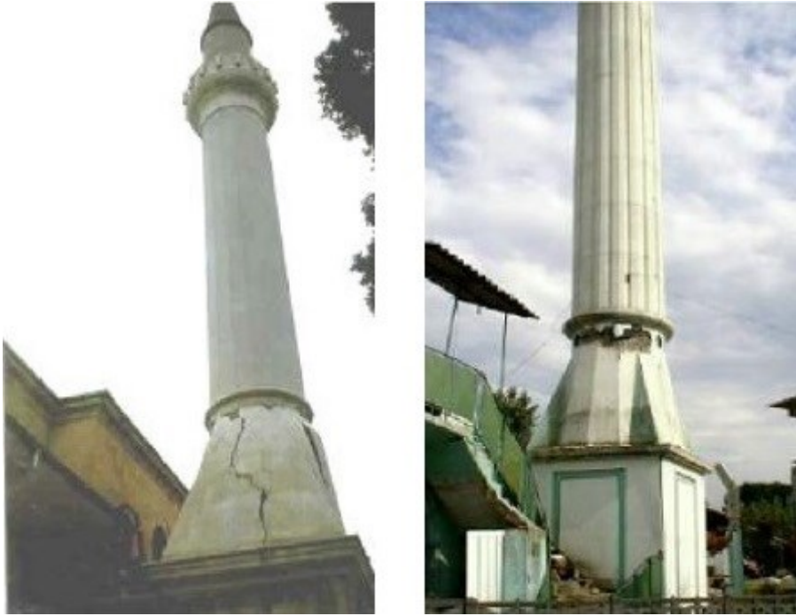
Figure 1.6: Damage to the transition segment (photos by (a) Firatand (b) Scawthorn).
