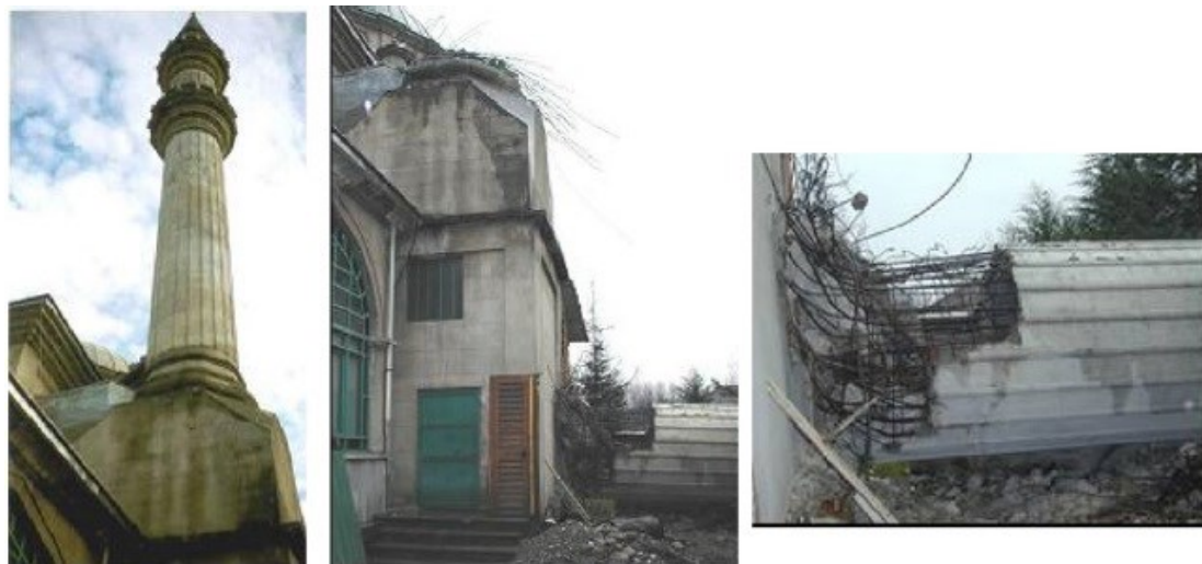
Figure 1.8: Minaret in Kocaeli after the August 17 earthquake (minor cracks) and November 12 earthquake (collapse).
